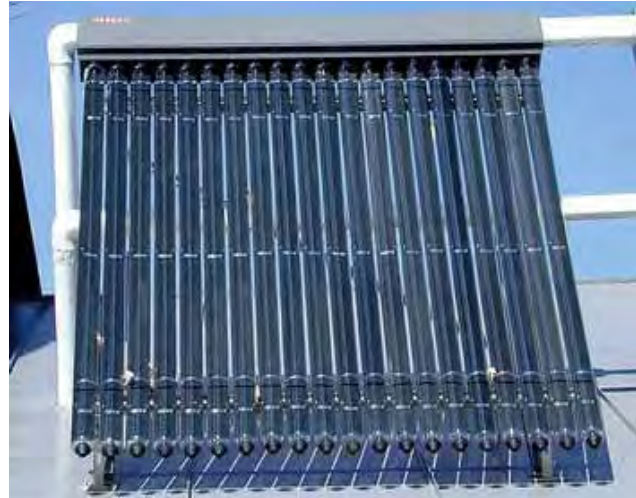
Evacuated Tube Solar Water Heating. Source: NREL Photo Exchange.
