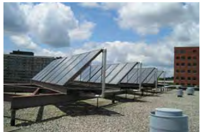
Solar hot water system on the top of the VA Hospital. Source: City of Ann Arbor.
