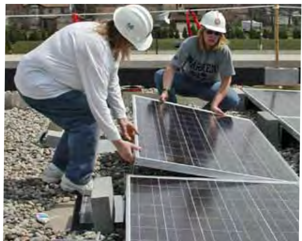
IBEW Training, Detroit. Source: GLREA.
