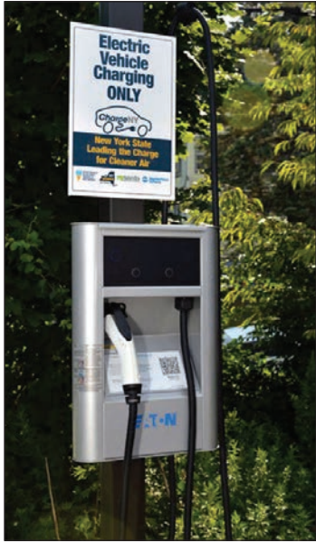
Example of Existing EV Charging Station (John Markowitz)
