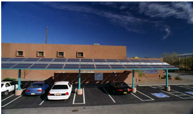
Figure 7: Solar PV Parking Canopy
