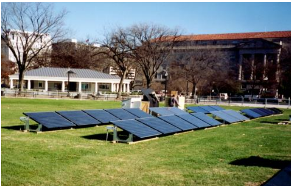
Figure 4: Ground-Mounted Solar Energy
