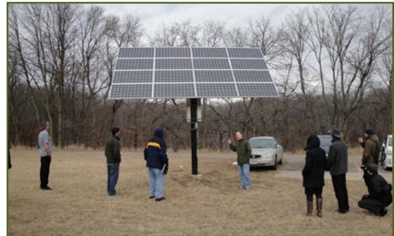
Ground Mount System, CERTs
