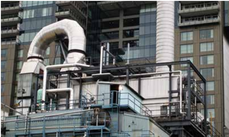
Seattle Steam Company heating district provides steam to 175 downtown businesses Source: Jason Brackins, Creative Commons
