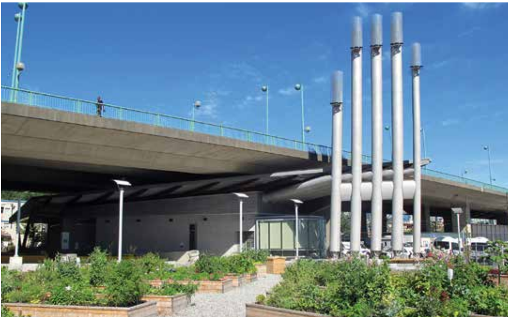
City of Vancouver Neighborhood Energy Utility serving Southeast False Creek neighborhood Source: Christopher Porter
