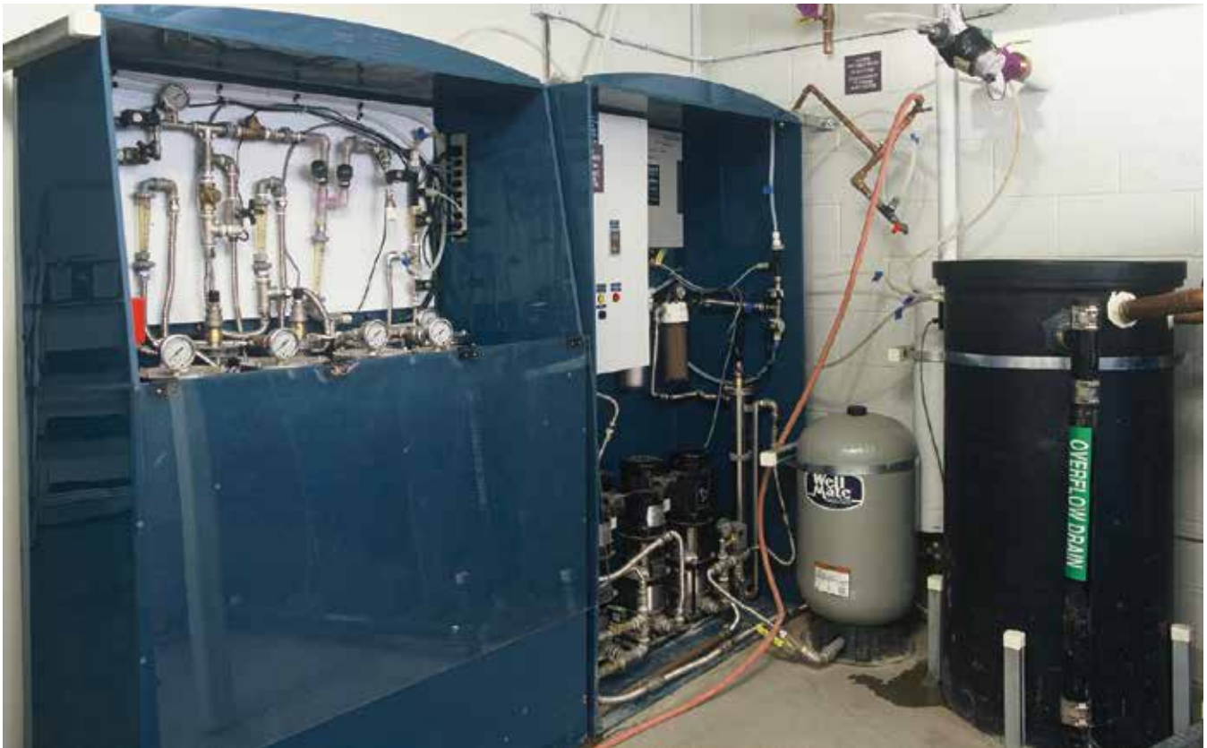
Graywater system in NRDC headquarters, Santa Monica, CA Source for image: Grey Crawford
