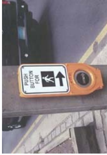
Accessible pedestrian push buttons indicate the WALK sign is lit through sound or other nonvisual signal. Push buttons should be located and signed according to MUTCD and PROWAG standards (MUTCD R10-4) (KAI)
