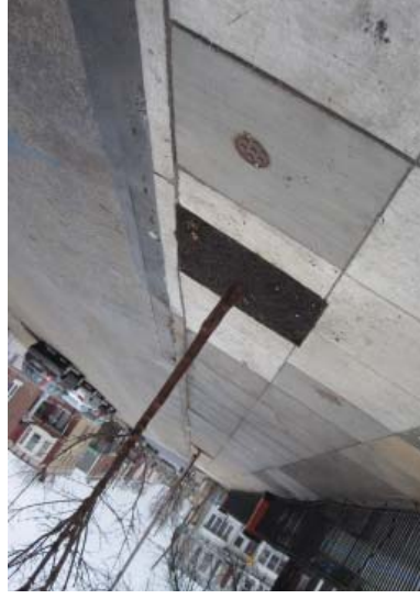
Tree pits should maintain adequate clear walking space and provide room for trees to grow without pushing up adjacent pavement such as this tree pit at the Hannity School at 56th and Webster.
