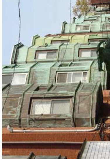
Bay windows may not extend onto or project over the minimum clear sidewalk width unless at least 10’ vertical clearance is maintained.
