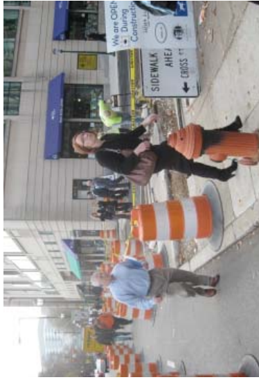
Construction within the public right-of-way or that extends into or over the sidewalk must provide the minimum clear sidewalk width (4.3.2) or an alternative accessible path.
