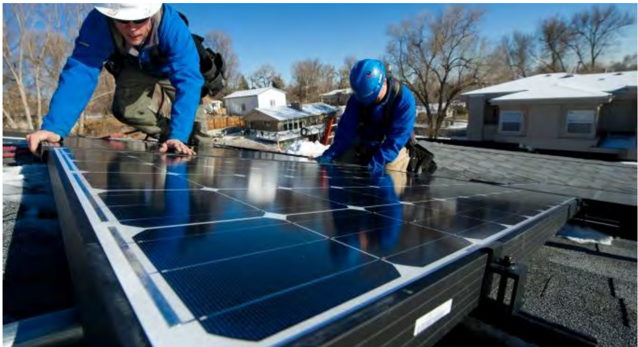
Rooftop solar installation. Photo courtesy of energy.gov
